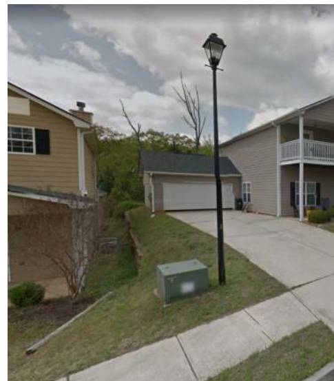
Photo 2. Retaining Walls, Drainage Problems.
